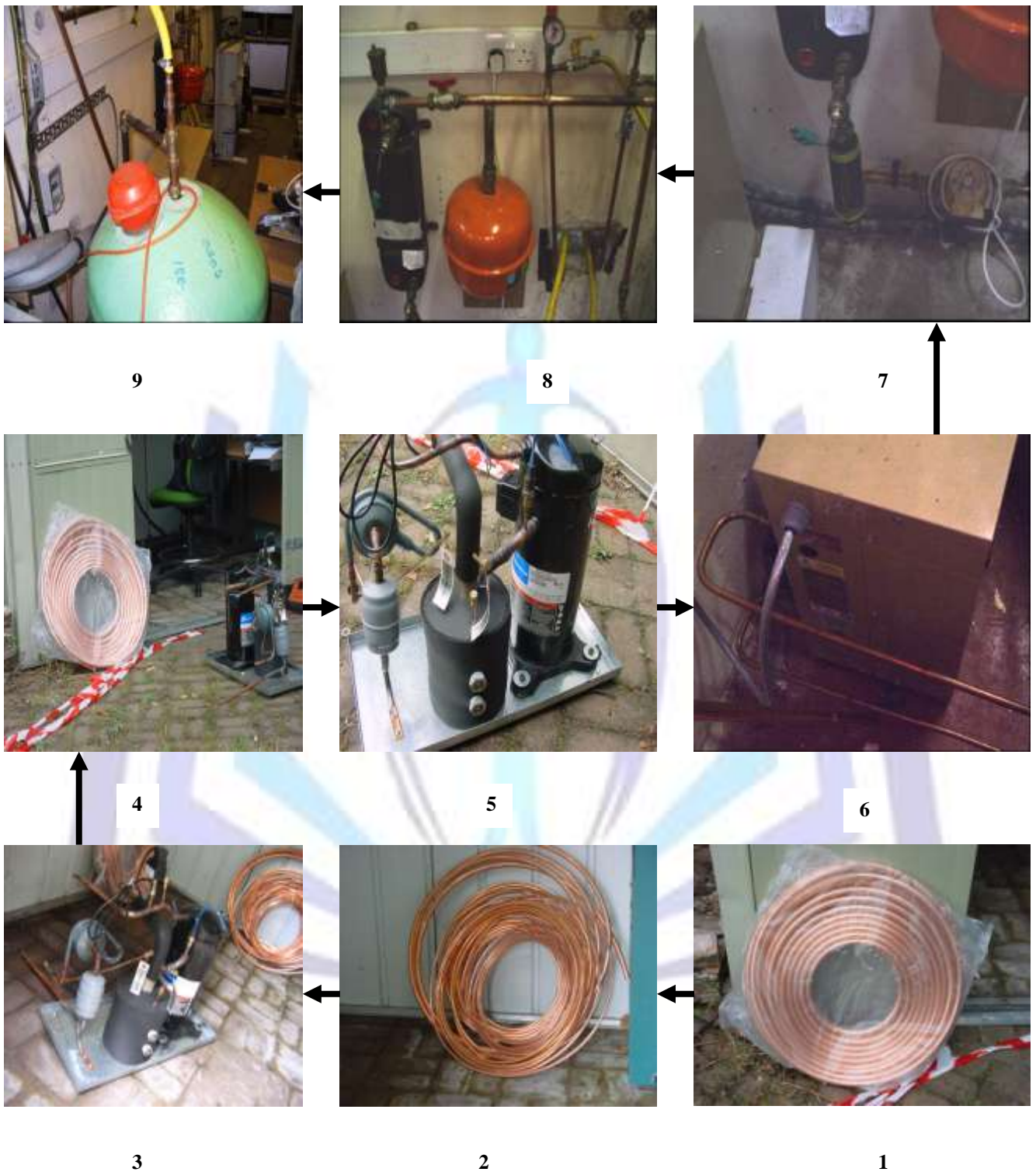
Figure 4 Showing preparation of coils (1-2), installation of heat pump (3-6) and connection of water supply system (water pump, flow metre, expansion valve and the boiler) (7-9)
