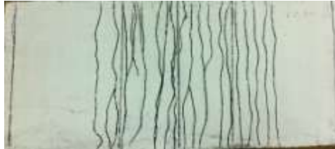
Figure 6 Failure patterns of ferrocement slabs
