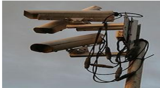
Fig. 1 Example of CCTV camera
